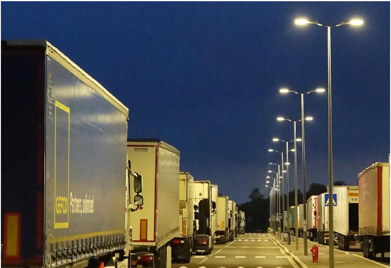
Eclairage des parkings, base logistique Eurologistic, Villabé, France – Luminaire Victoria © EAS solutions
